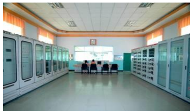
Figure 2. pump station control room
